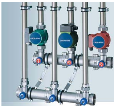
Start with pumps
